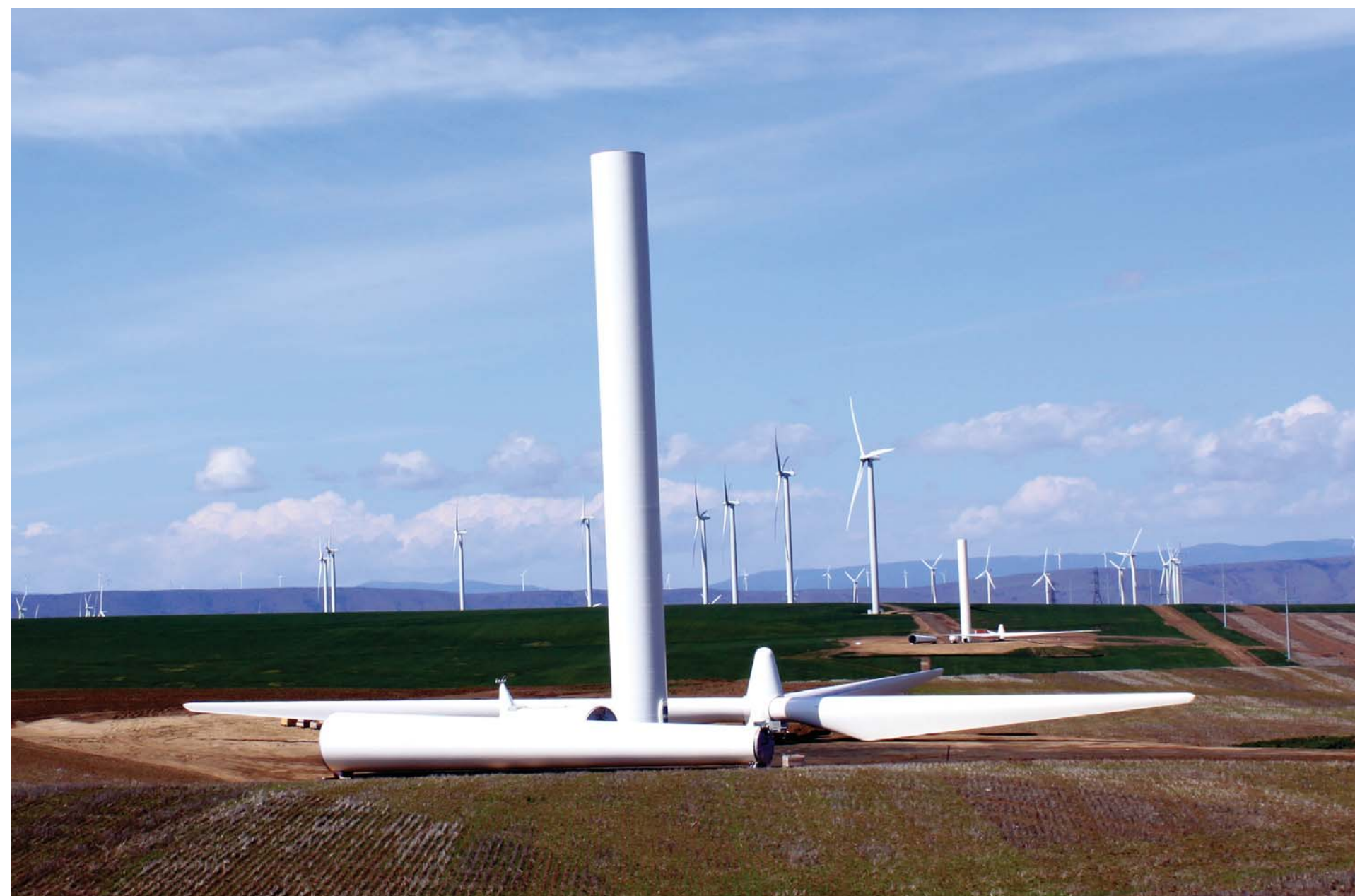
The 450MW Biglow Canyon Wind Farm under construction in Oregon. Source: Ted Timmons (2009)
